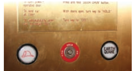
Unique to Seattle: A special elevator button to push in case of an earthquake.
